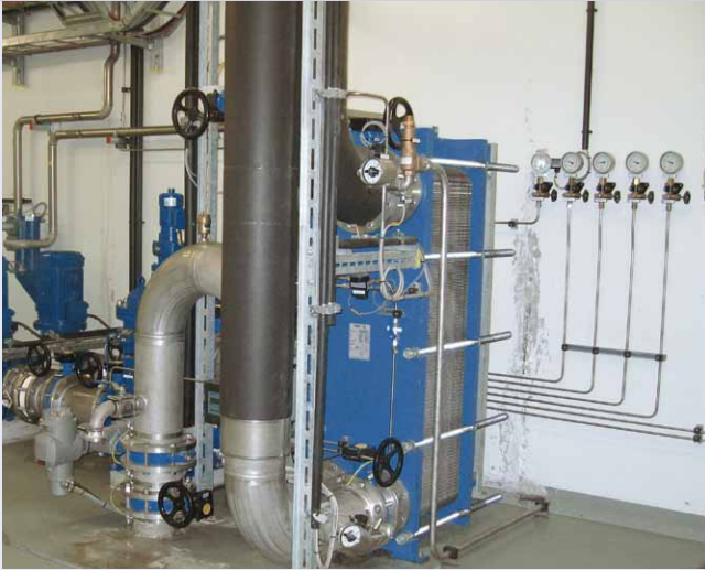
Hydraulic oil cooling in power plant.
