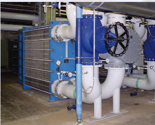
Cooling of laser welding plants in automotive production.
