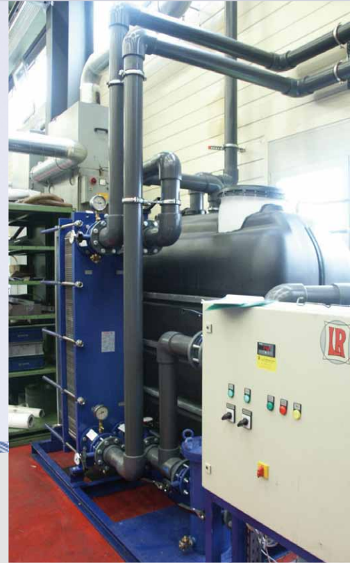
Cooling of lubricating oil for extruding presses.
